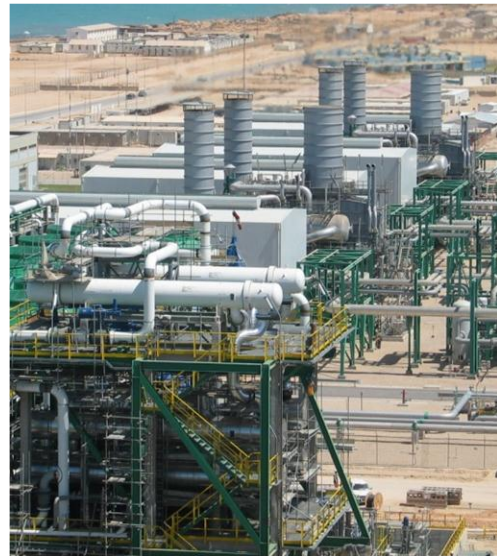
Fig. 3. Natural gas compressor station - Ecompi
